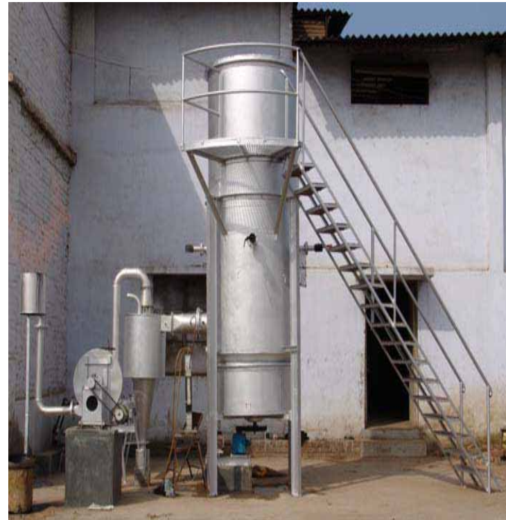
Producer gas system installed in an industry near Anand (Gujarat) for chicory roasting
